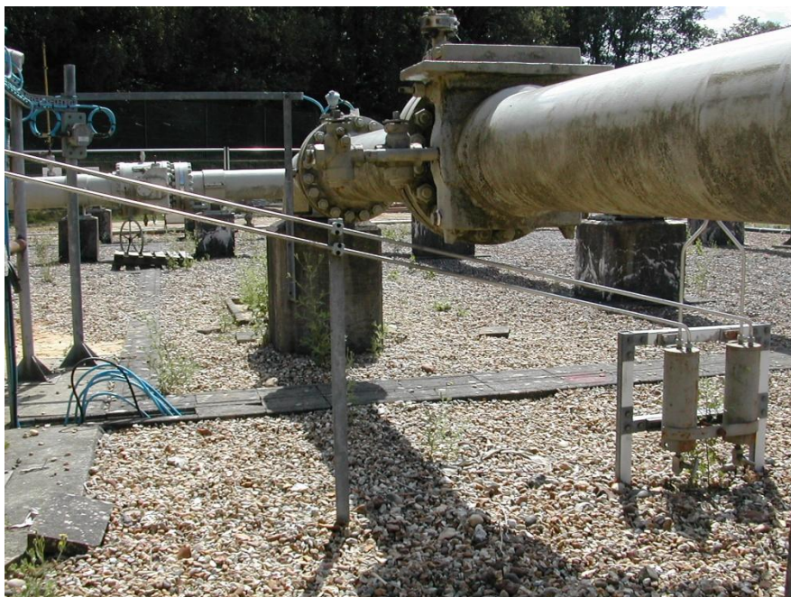
Figure 4.8 – Transmitter Impulse Lines and Catchpots
