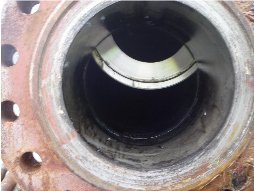
Figure 5.2.5 – Orifice Plate Position (Counter Reading 99960)
