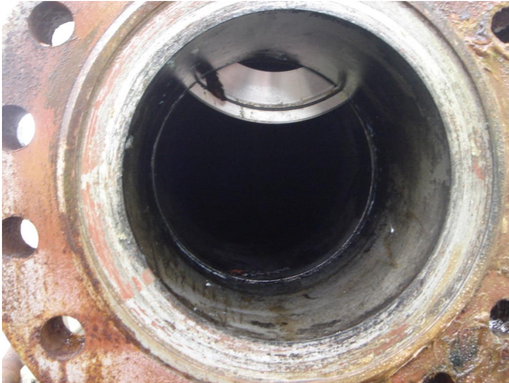
Figure 5.2.6 – Orifice Plate Position (Counter Reading 99940)
