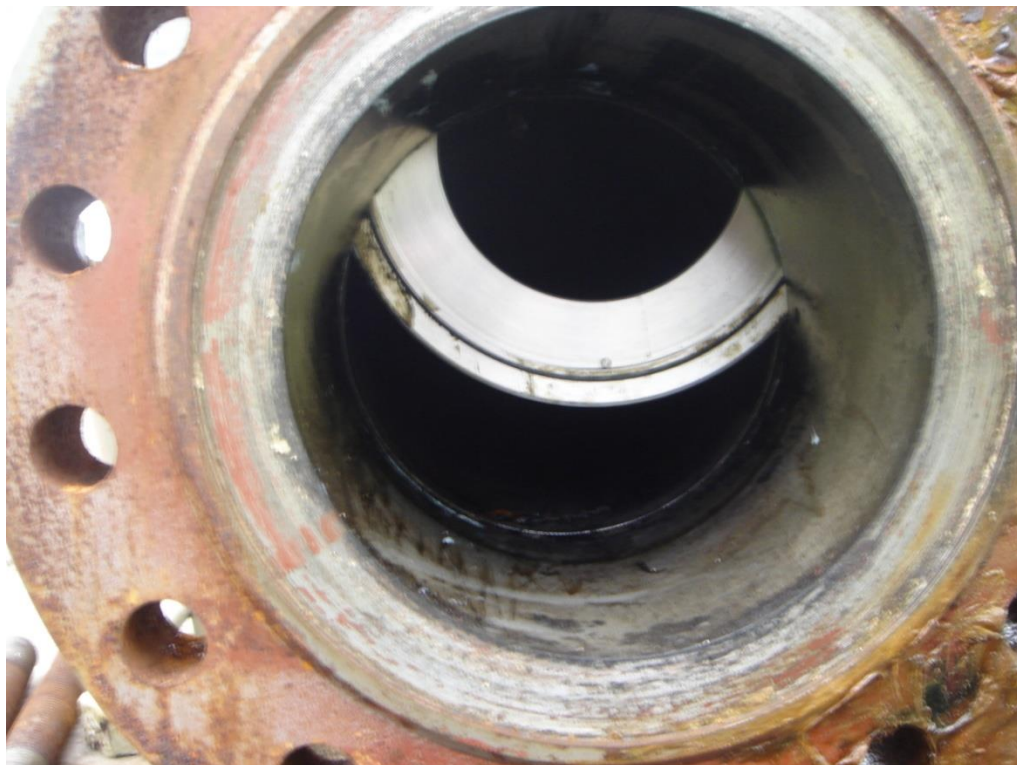
Figure 5.2.4 – Orifice Plate Position (Counter Reading 99970)
