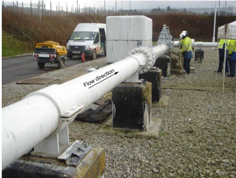
Figure 7. Photograph of the site and pipe layout near the metering location
