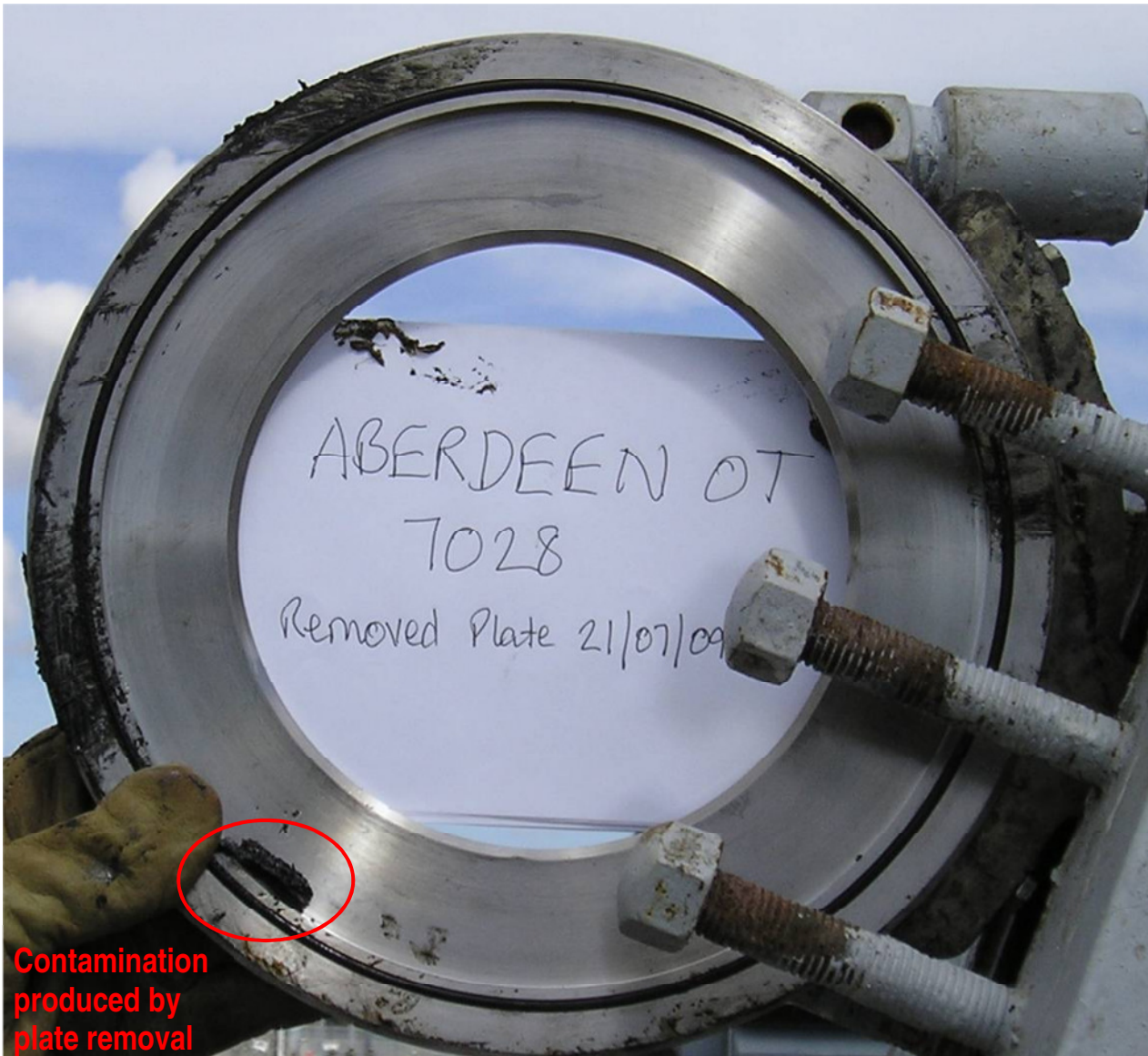
Figure 21 - Orifice Plate 050/4 Removed on 21st July 2009 (Downstream)
