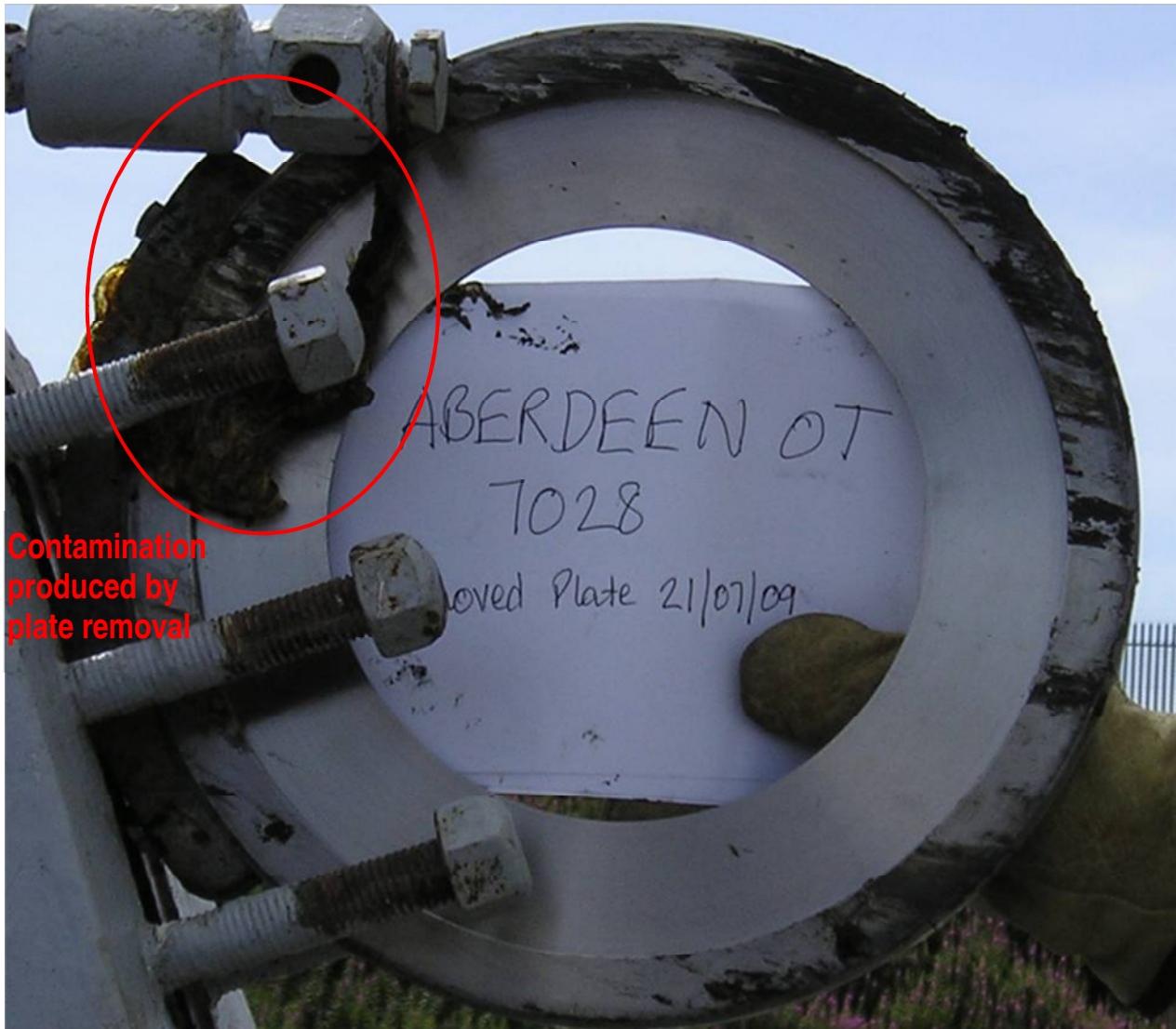
Figure 20 - Orifice Plate 050/4 Removed on 21st July 2009 (Upstream)
