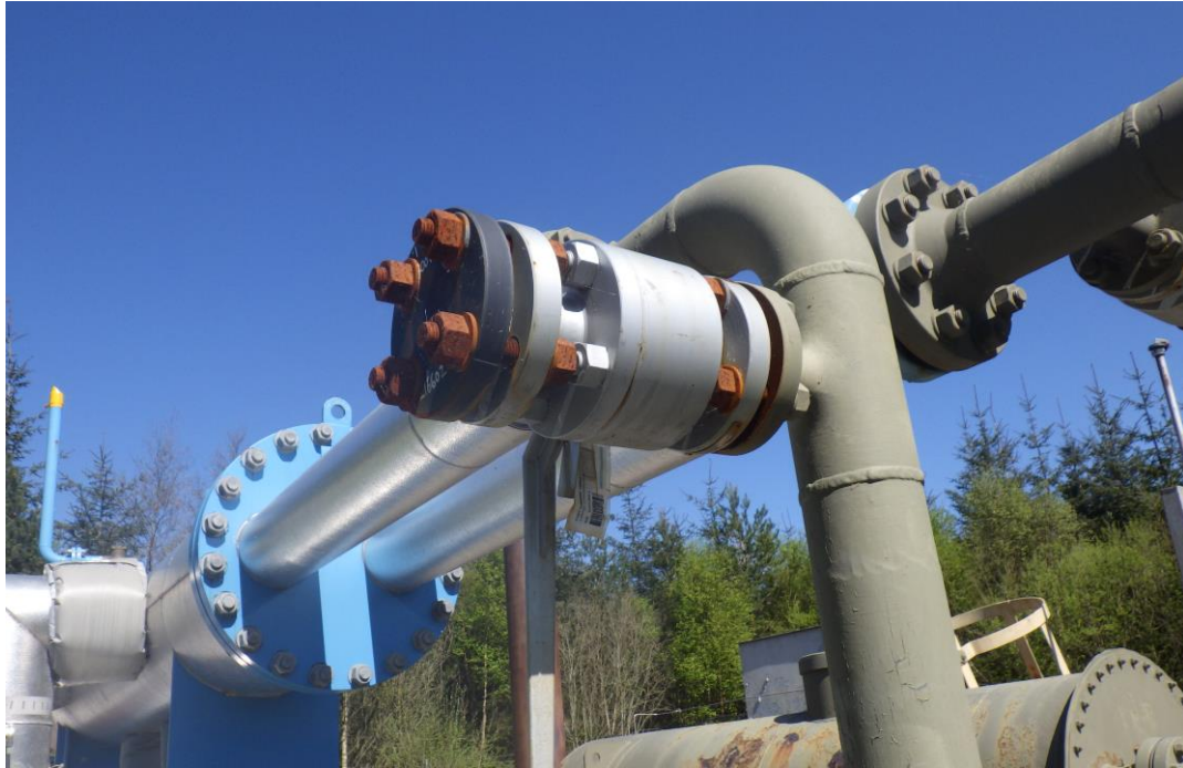
Figure 4: Pro-Heat Immersion Tube Preheater at Lochmaben (Existing Water Bath Heater in background)
